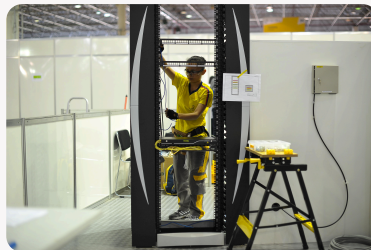
Information Network Cabling
